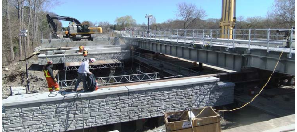
Sliding the new GO train bridge (between Main Street & Kennedy Road) into place.
